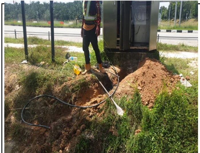
cable already inside the feeder pillar
