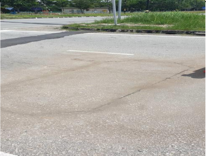
loop detedtor completed
