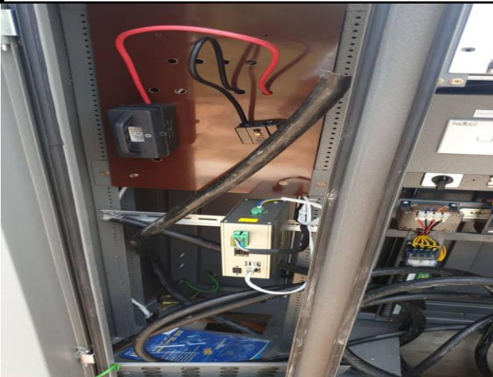
power cable inside the controller
