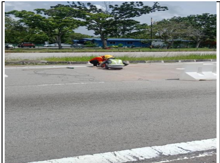
lay cable loop detector
